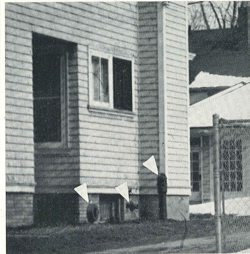
Sprinkler alarm bell, fire department siamese and post indicator valve at side of Toledo nursing home, are unobtrusive yet readily available.
